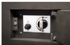
Concealed Control Panel
