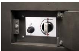
Concealed Control Panel
